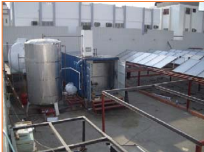
Picture: 5m 3 system with 140m 2 Flat collectors in Jeddah, Saudi Arabia
